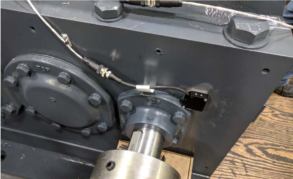
Figure 17 – Vibration sensor on split face of housing cover with 45 degree edge at 11 o'clock and cable to top left
