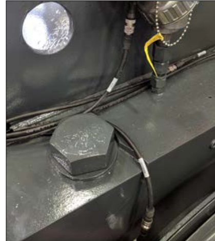
Figure 39 – Cable routing on top of split bolt ledge.
